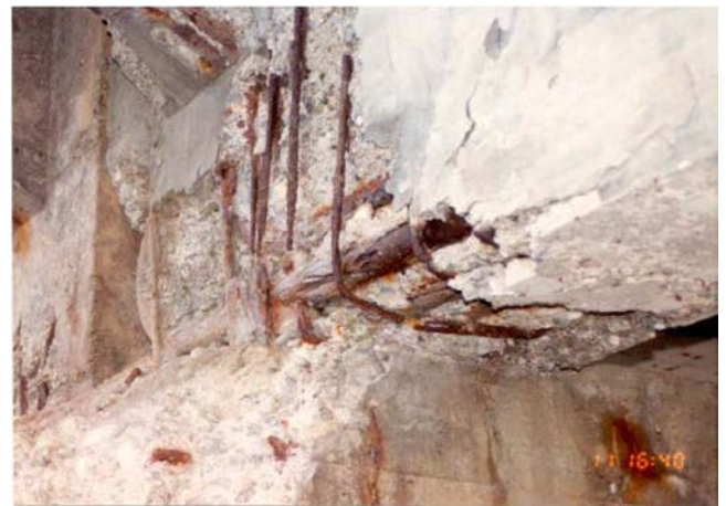
Fig. 1—Example of severe reinforcing steel deterioration due to corrosion in a reinforced concrete beam (courtesy of the Ministry of Transportation of Quebec).
