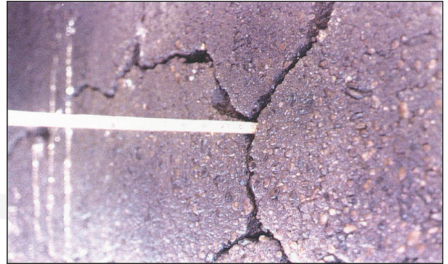
Fig. 1—Wide cracks in concrete as a result of AAR (width of the order of 1 in. [25 mm] in certain areas).
