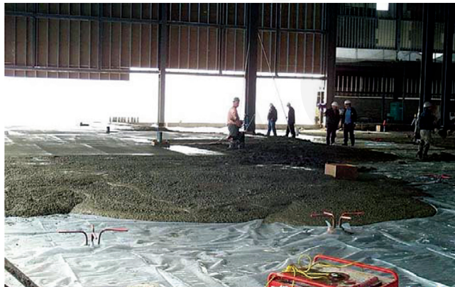
Fig. 1.1a—Installation of G-SFRC slab (pile-supported ground slab) (courtesy of Bombardier Aerospace Inc.).
