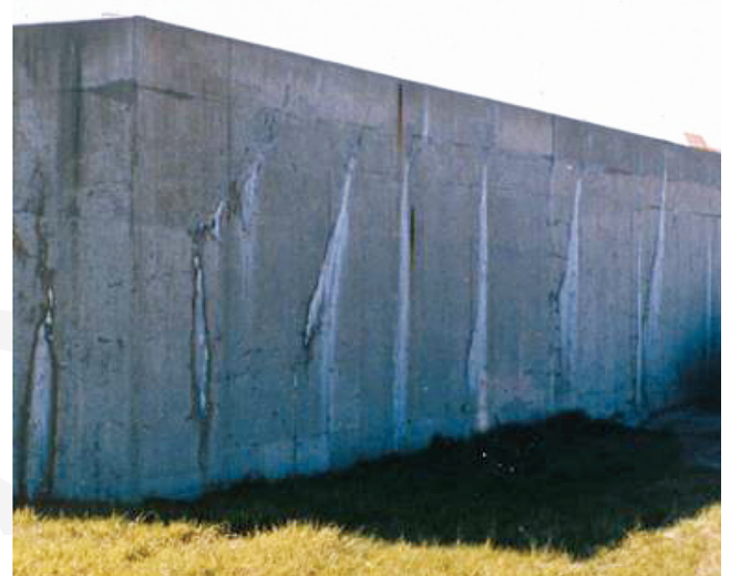
Fig. 1—Vertical cracking at the walls of a liquid containment tank.
